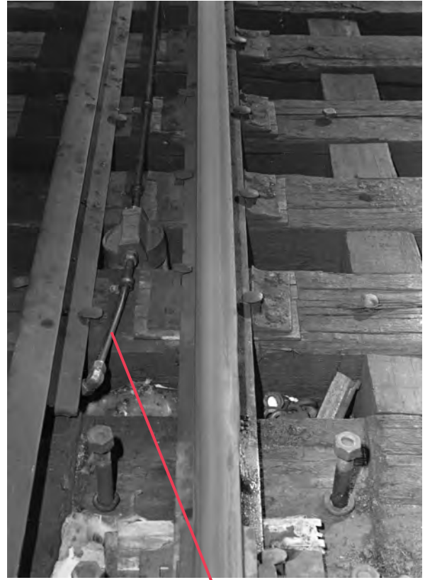
Protectowire Linear Heat Detector within tubing
